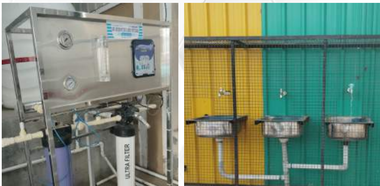
Image: UV Treatment Plant supported by KVB
